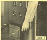
Main Disconnect Switch
